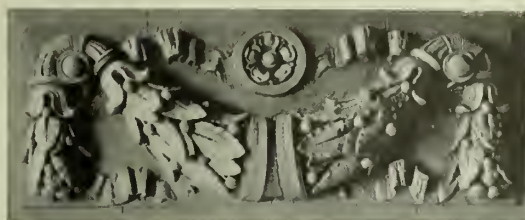
DETAIL BY ROUSE & GOLDSTONE, ARCHITECTS. New York Architectural Terra Cotta Company, Makers.
